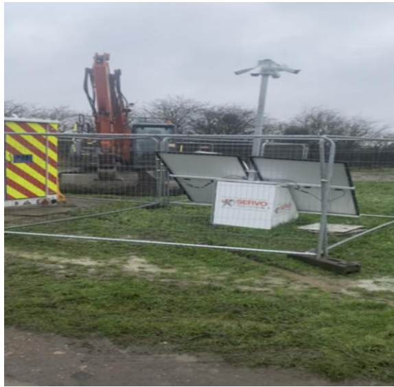
P15 Compound – Stand alone CCTV facing over compound , Fencing 1.8 -2 m Security Fencing
