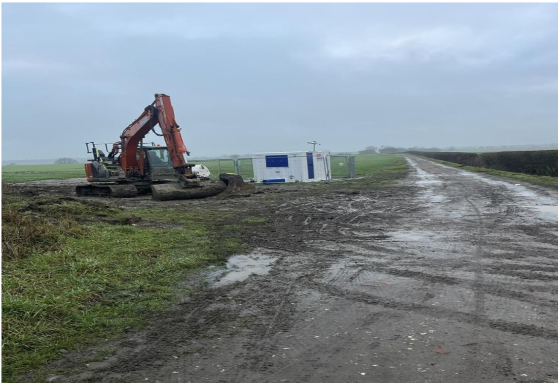
P3 21.1.26 (Compound placed immediately after blind bend)
